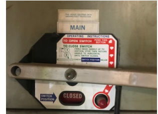
Exterior Service Disconnect
