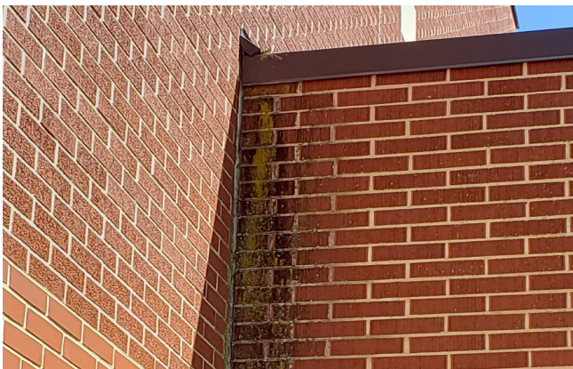
SUNRISE - Roof water damage to wall
