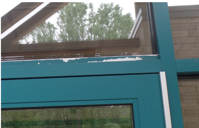
SAWYER - Door frame finish failing
