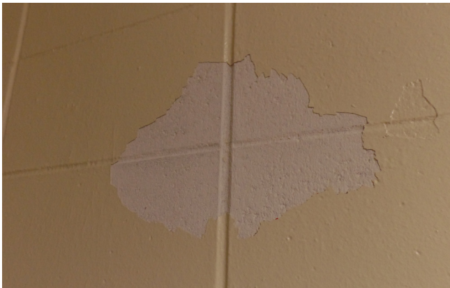
MIDDLE SCHOOL - Peeling paint on walls
