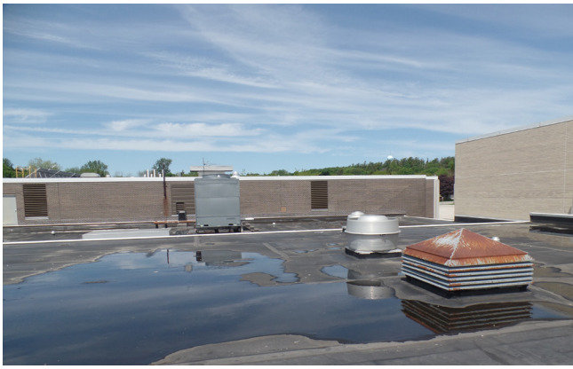
MIDDLE SCHOOL - Ponding water on roof / rusting roof vents
