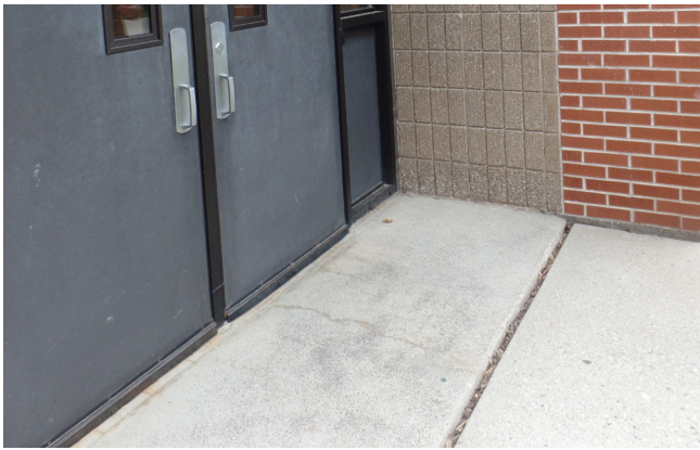
SUNSET - Stoop slab / sidewalk settling causing unsafe conditions.
