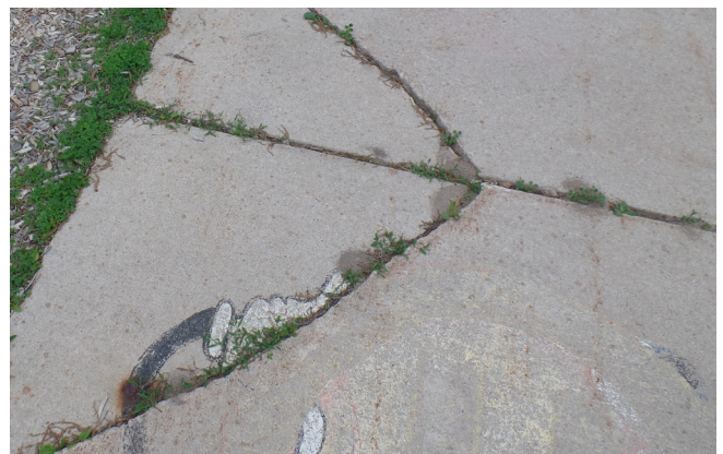
SAWYER - Cracked pavement / sidewalks
