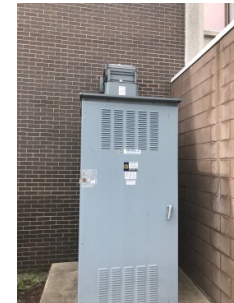
Exterior Service Disconnect
