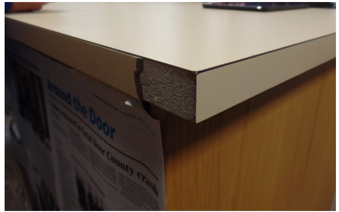
MIDDLE SCHOOL - Millwork showing signs of wear
