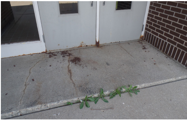
MIDDLE SCHOOL - Failing door / frame and uneven stoop / sidewalk slabs
