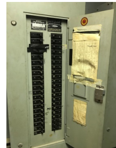
Electrical Panel - Westinghouse
