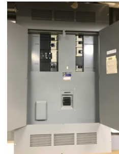
Electrical Main Panelboard
