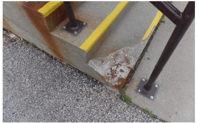
SUNSET - Deteriorating exterior concrete
