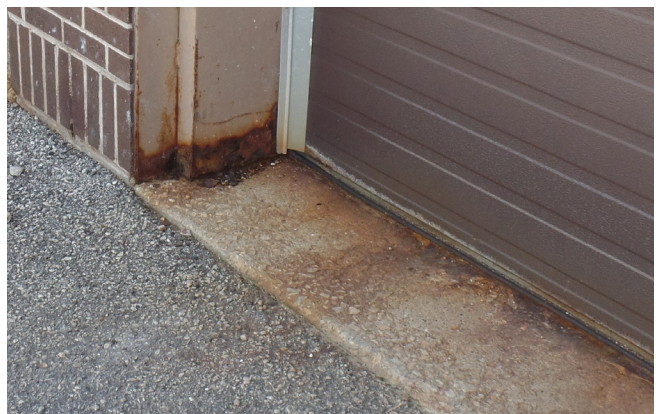
HIGH SCHOOL - Rusting door frames
