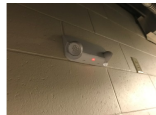
Emergency Lighting – Battery Unit
