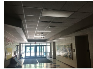
Corridor Acrylic Light Fixtures
