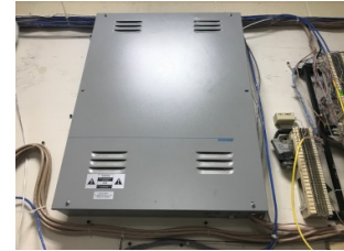
Paging System Equipment
