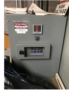
High School Automatic Transfer Switch
