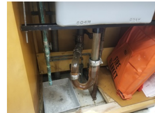
HS Lab Drains
