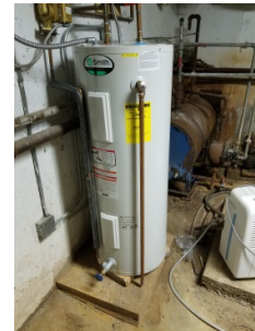
Sunrise Basement Water Heater
