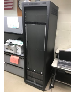
Paging Headend Equipment
