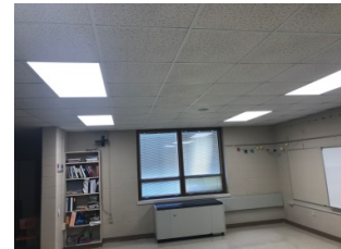
Typical Fluorescent Acrylic Lighting
