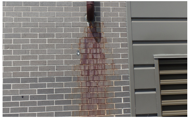
MIDDLE SCHOOL - Penetrations through wall rusting and staining masonry
