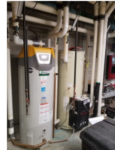
HS Water Heaters
