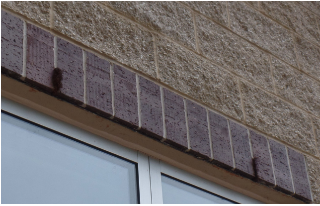
SAWYER - Incorrect masonry weeps / vents
