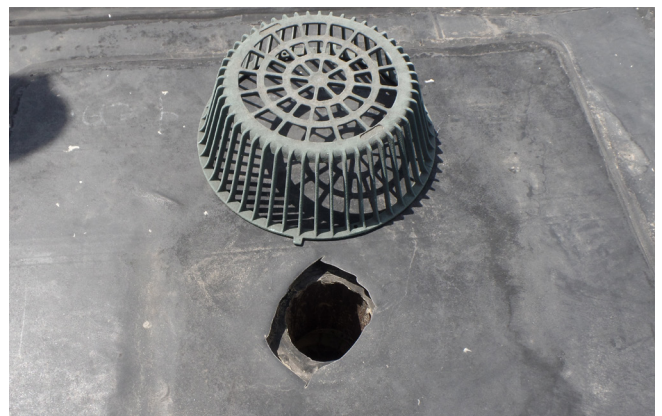
MIDDLE SCHOOL - Improper roof drain installation
