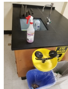
Emergency Eye wash
