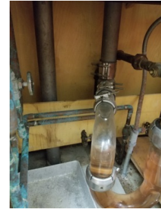
Domestic Water Valves
