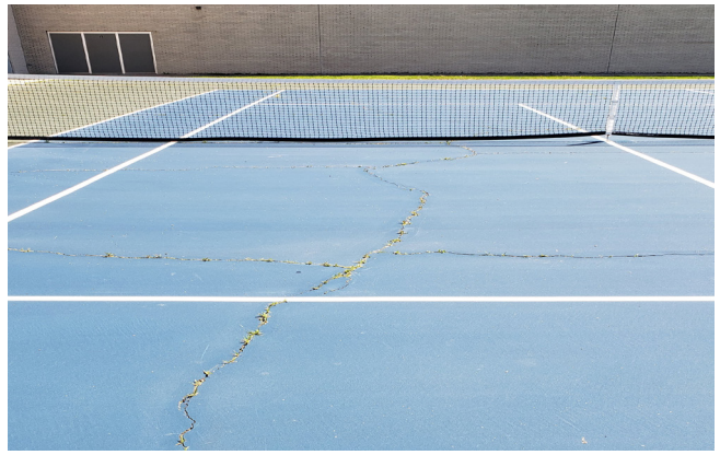
HIGH SCHOOL - Tennis court pavement cracked and failing
