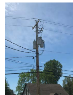
Pole Mounted Utility Transformer
