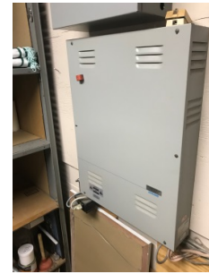
Paging System Equipment
