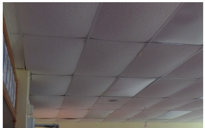
SUNSET - Ceiling tiles damaged / sagging due to high humidity
