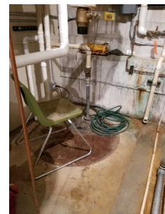
Sump Pump - Addition
