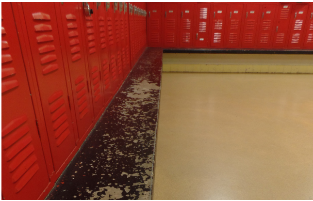
HIGH SCHOOL - Locker room equipment, lockers and flooring showing wear / failing.
