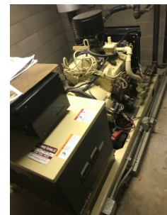
Emergency Generator (HS and MS)
