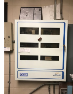
Fire Alarm Control Panel
