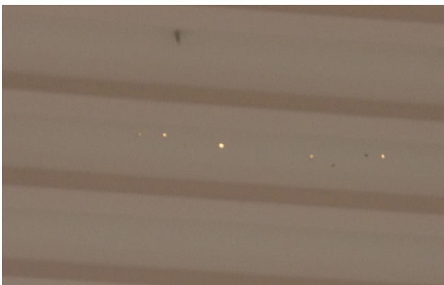
HIGH SCHOOL - Random holes in roof deck at wrestling / work out room
