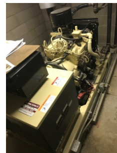
Emergency Generator (HS and MS)
