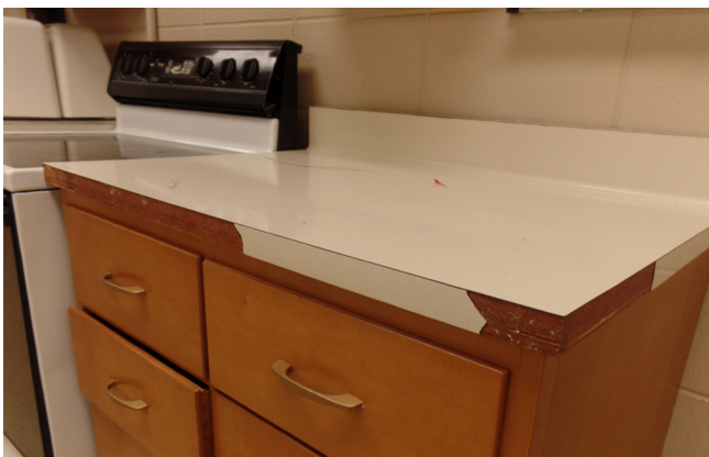
HIGH SCHOOL - Millwork failing / showing wear
