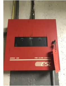
Fire Alarm Control Panel
