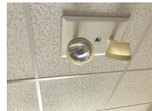
Emergency Lighting – Battery Unit
