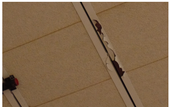
MIDDLE SCHOOL - Rusting / failing paint on ceiling beams in gym
