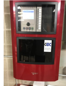
Fire Alarm Control Panel (HS & MS)
