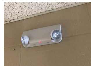
Emergency Lighting – Battery Unit
