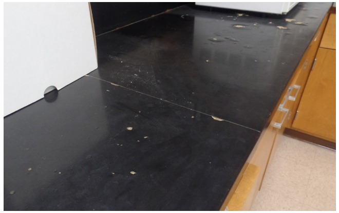
MIDDLE SCHOOL - Damaged millwork / counter-top
