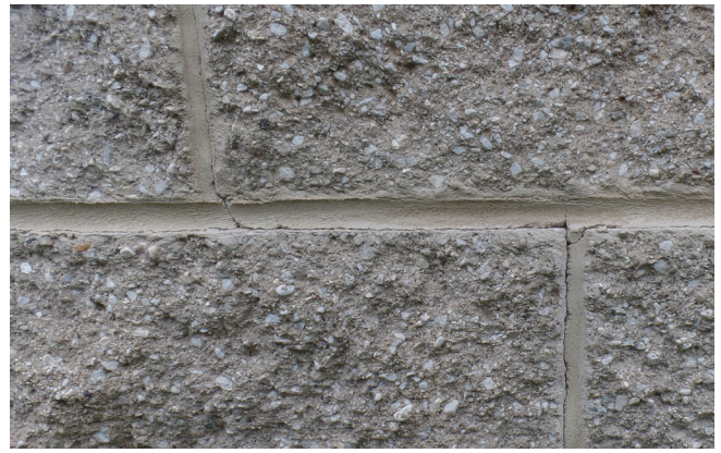
SAWYER - Cracked masonry mortar joint
