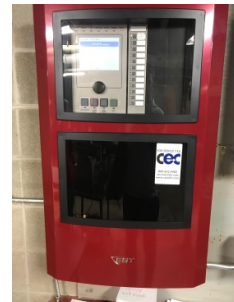
Fire Alarm Control Panel (HS & MS)
