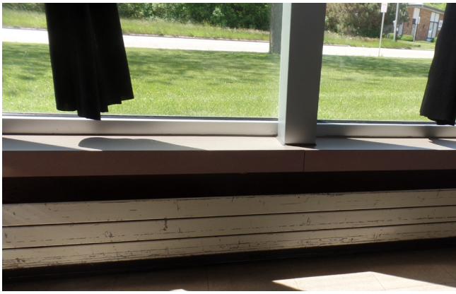
HIGH SCHOOL - Radiators showing signs of wear
