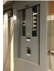
Electrical Main Service Panelboard
