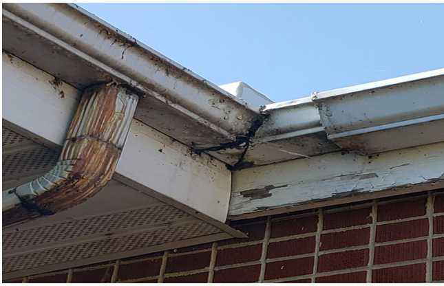
SUNRISE - Failing gutter / downspout / eaves
