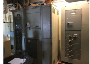
Electrical Main Switchboard
