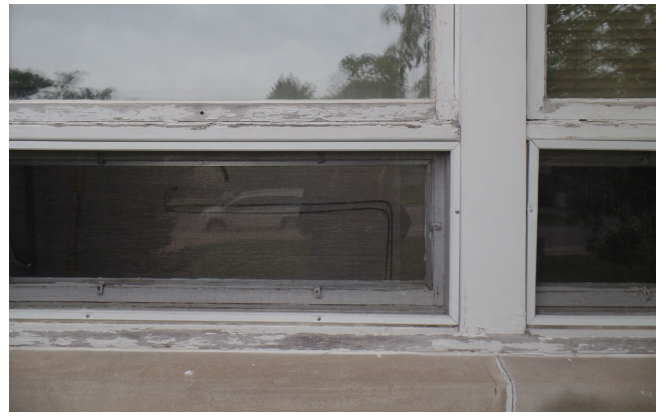
SUNSET - Failing windows
