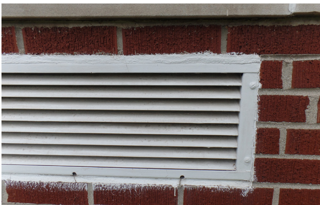
SUNRISE - Poorly fit / sealed louvers and vents
