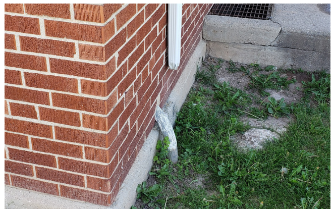
SUNRISE - Downspouts not connected/ improper site drainage
