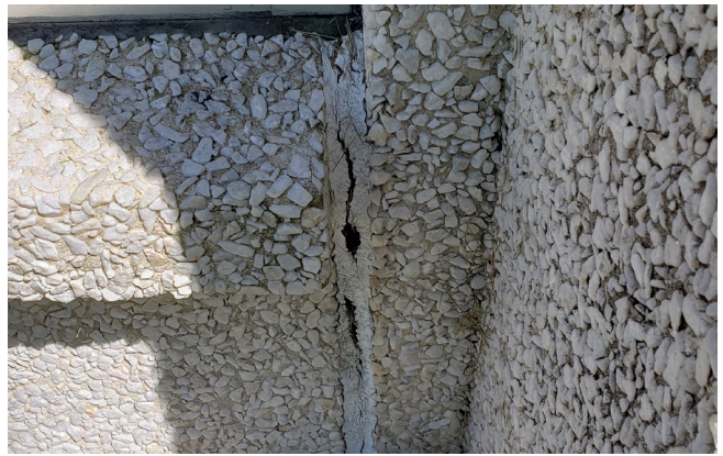
HIGH SCHOOL - Failing sealant joints
