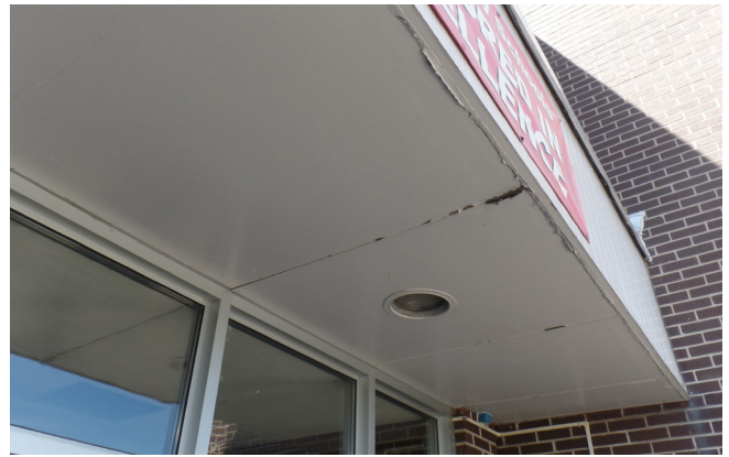
MIDDLE SCHOOL - Failing soffit / asbestos materials
