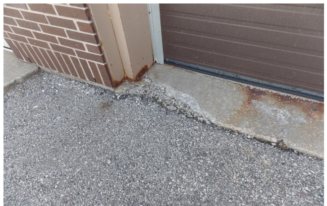
HIGH SCHOOL - Concrete failing
