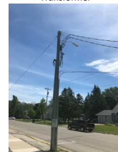
Overhead Electrical Service
