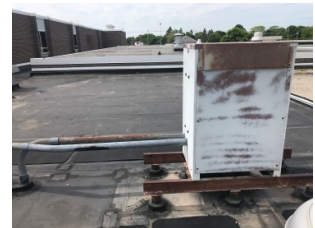
Roof Mounted Transformer
