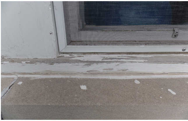
SUNSET - Failing / missing paint
