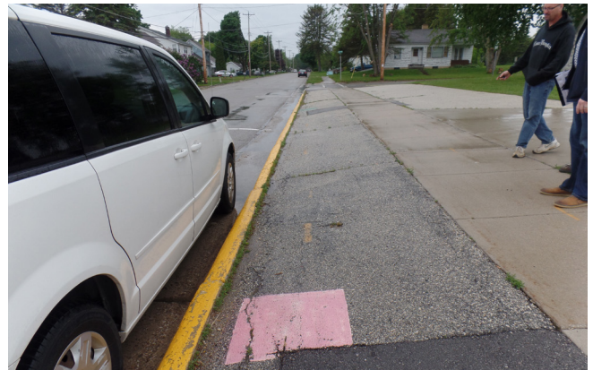
SUNRISE - Inaccessible (ADA) / unsafe pavement at student pickup / drop-off area
