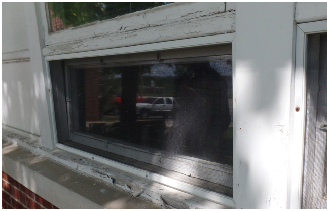
SUNRISE - Failing windows
