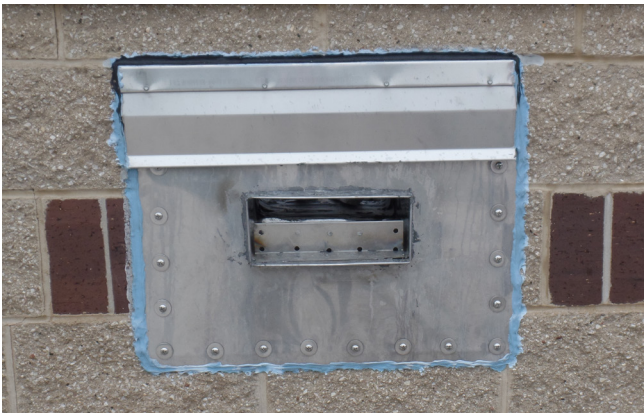
SAWYER - Poor scupper patch at parapet
