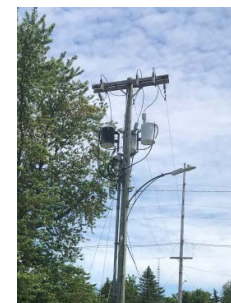
Pole Mounted Utility Transformers
