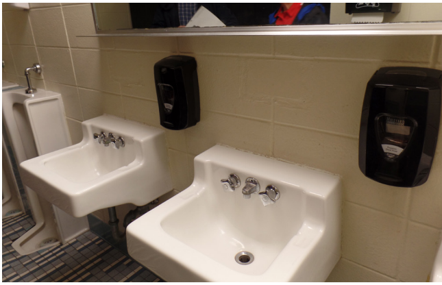
MIDDLE SCHOOL - Inaccessible (ADA) restroom fixtures and accessories
