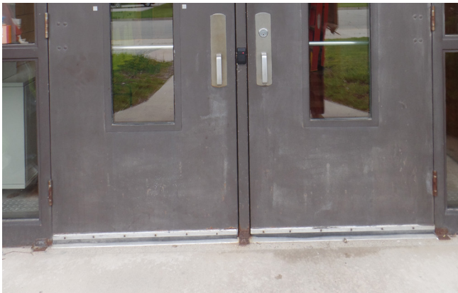
SUNRISE - Rusting / failing door frames
