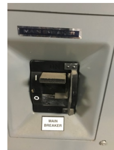
Electrical Main Service Disconnect Switch
