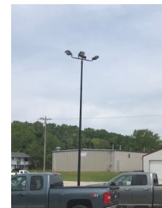
Parking Lot Pole Lighting
