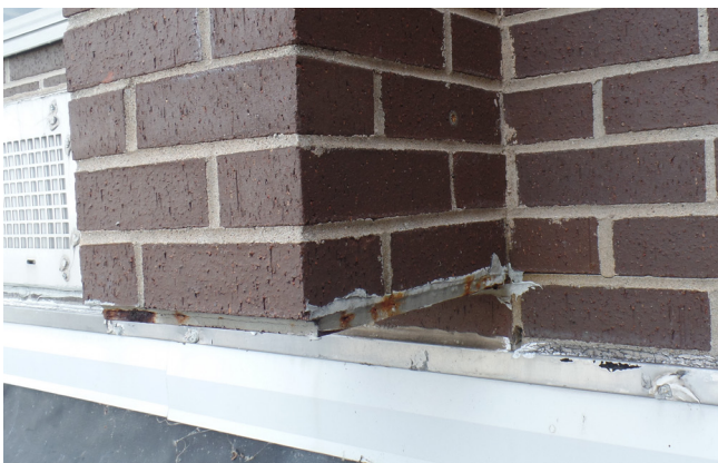
MIDDLE SCHOOL - Rusting masonry supports
