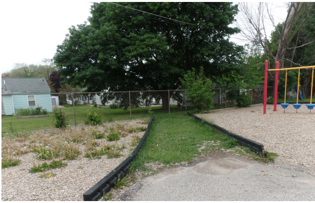
SUNSET - Poor site drainage
