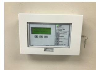
Fire Alarm Annunciator Panel
