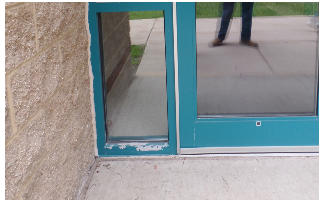
SAWYER - Door frame finish failing
