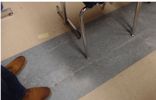
MIDDLE SCHOOL - Flooring failing / peeling away from concrete
