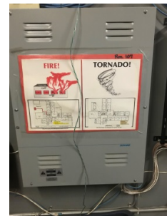
Paging System Equipment
