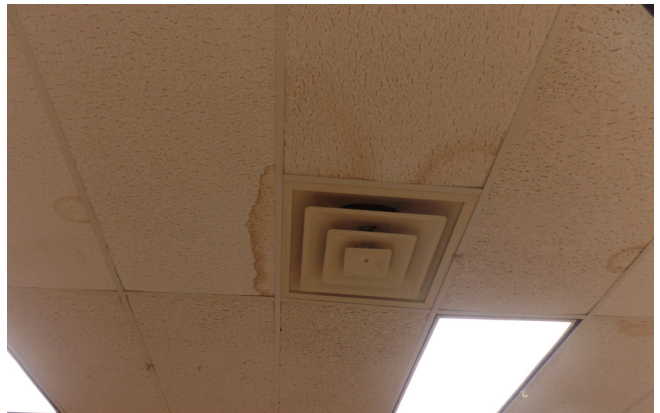
MIDDLE SCHOOL - Stained ceiling tiles
