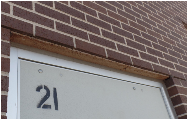
HIGH SCHOOL - Rusting masonry lintels
