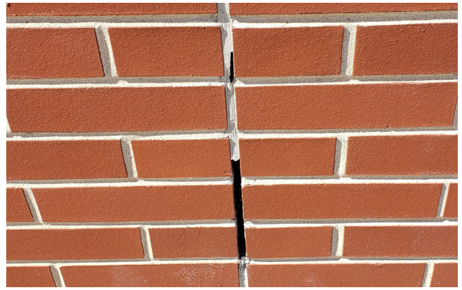
SUNRISE - Missing masonry mortar
