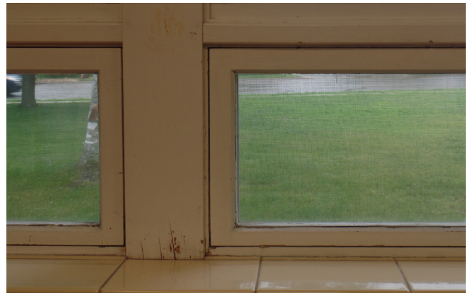
SUNSET - Failing windows
