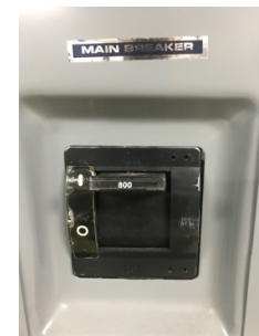
Exterior Service Disconnect Switch
