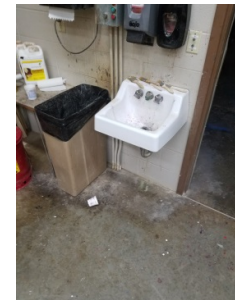
MS Shop Lavatory
