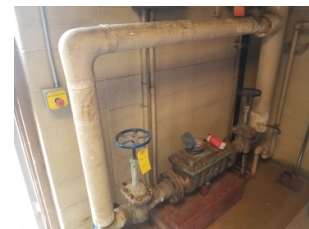
MS Water Meter
