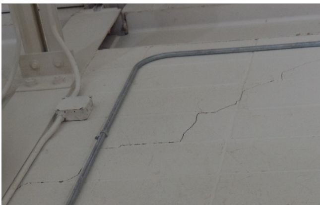
HIGH SCHOOL - Cracked block wall
