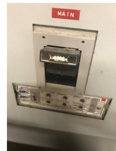
Electrical Main Service Disconnect Switch
