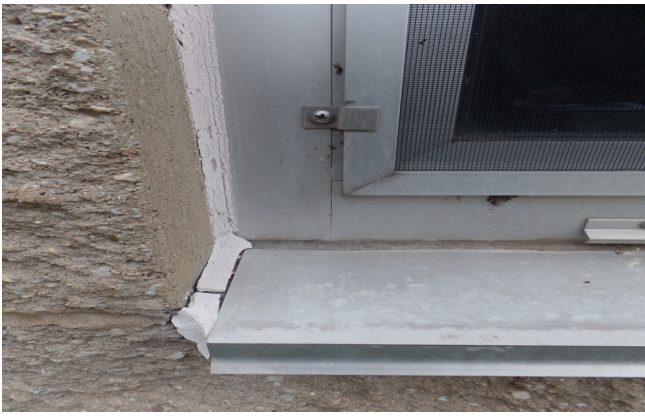
SAWYER - Window caulk / sealant failure
