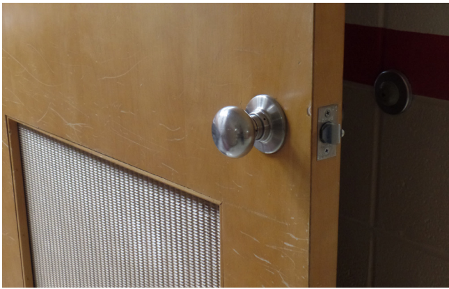
MIDDLE SCHOOL - Inaccessible door hardware (ADA)
