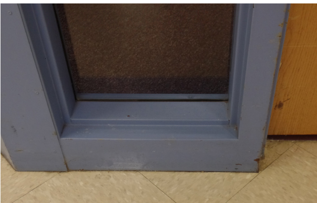
SAWYER - Finish showing wear on doors and frames
