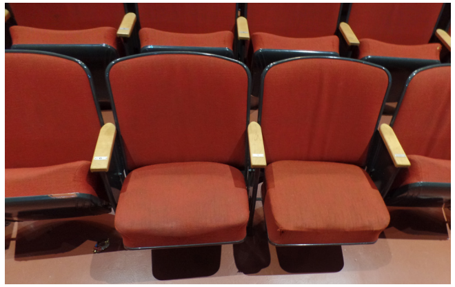
HIGH SCHOOL - Auditorium seating showing wear
