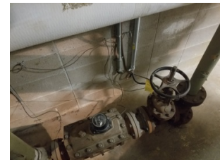
HS Water Meter
