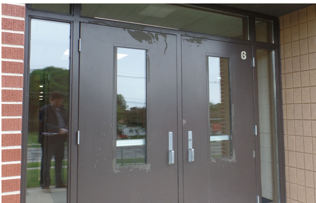
SUNSET - Door finish failing
