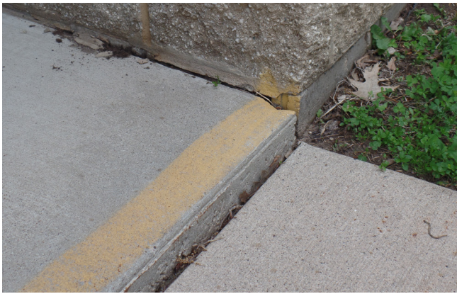
SAWYER - Door stoop / sidewalk settling trip hazard
