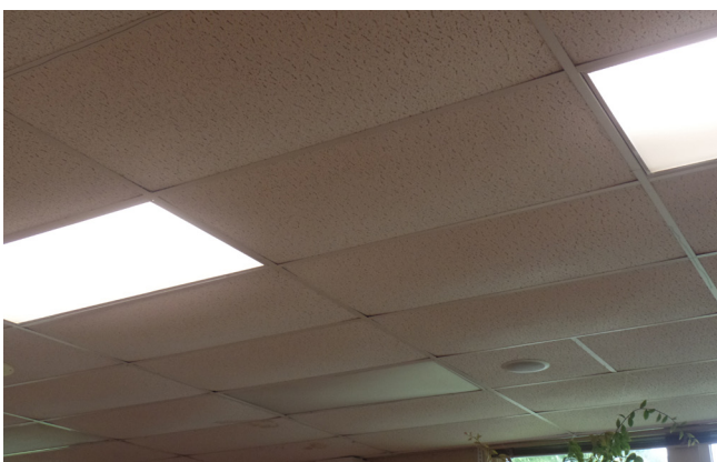
SUNRISE - Sagging ceiling tiles due to excessive humidity
