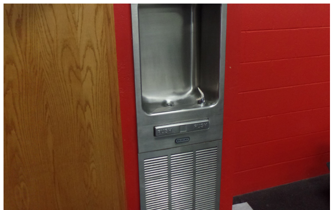
HIGH SCHOOL - Inaccessible drinking fountain (ADA)
