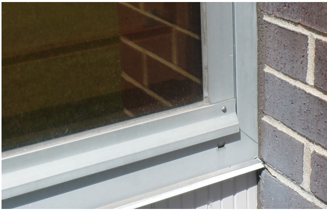
MIDDLE SCHOOL - Failing sealants at windows and louvers
