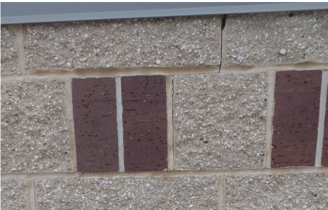
SAWYER - Cracked masonry at parapet
