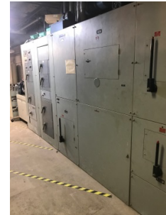
Electrical Main Switchboard
