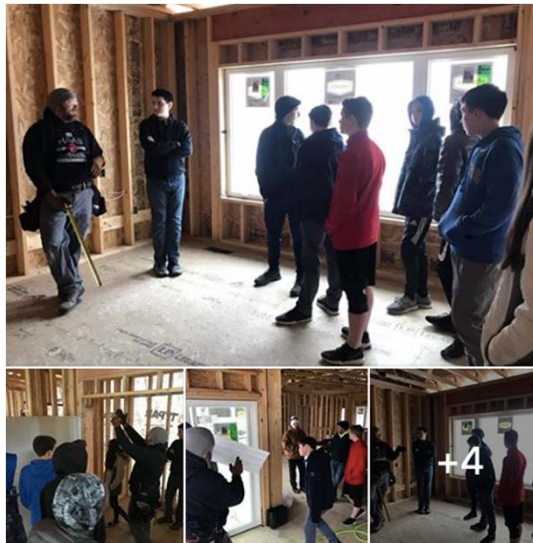
Mitchell Shield, a graduate of Sturgeon Bay High School and Territory Manager for Weather Shield Windows & Doors, came to the High School Home Construction Project job site last week. He brought with him Joseph Dowden from Technical Support to show how to install Weather Shield windows.
